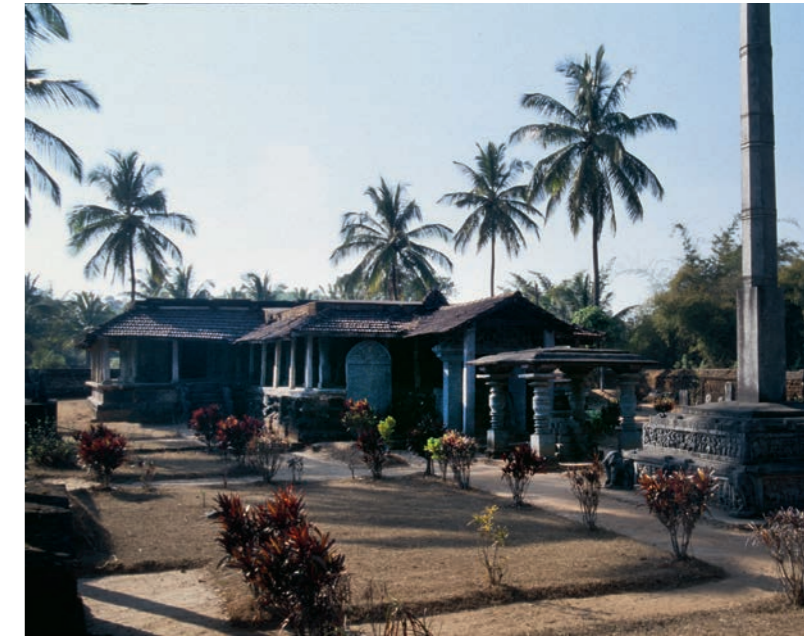
Plate 5: The basement of the entrance hall of the Panca Basadi at Humcha has been made of the locally available but soft and porous laterite, which is not a durable construction material.
