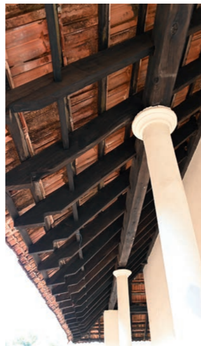
Plate 3: The roofs of the local Jaina temples, such as that of the Parshvanatha Temple at Venur, have been made of a wooden substructure covered with terracotta tiles.
